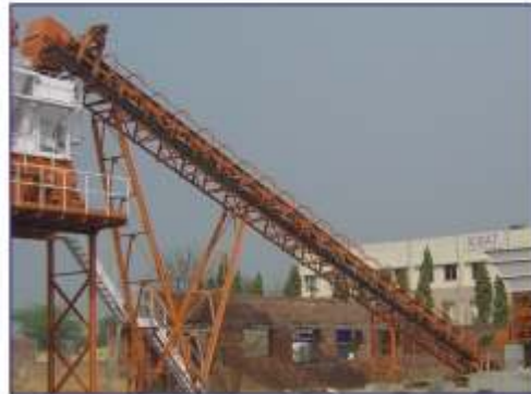
AGGREGATE CONVEYOR : Aggregate charging by belt conveyor.
